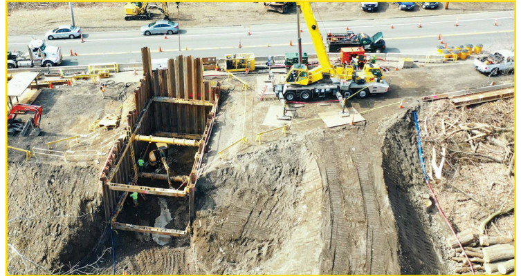
This work site in Ansonia shows just a few potential hazards Brennan employees face on the job, from heavy equipment moving around the workers, to deep trenches and uneven ground.
